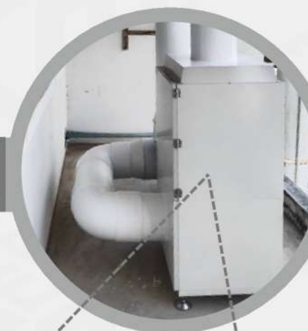
Activated carbon filter
